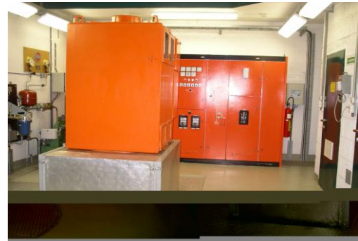
Generator, Sagfossen, Siljan
